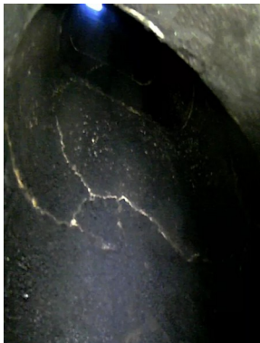
Flue Scan 1 Foot
